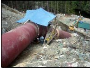
Penstock into the Power House
